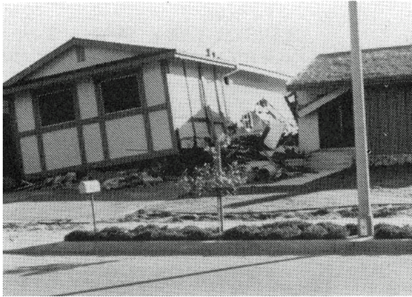
Building has collapsed, partially collapsed, or moved off its foundation. Condition: UNSAFE
