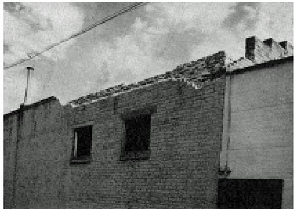
Obvious parapet or other falling hazard. Condition: AREA UNSAFE
