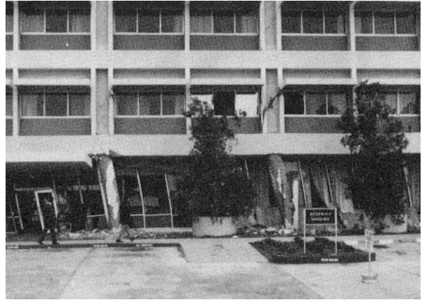
Building or any story is significantly out of plumb. Condition: UNSAFE
