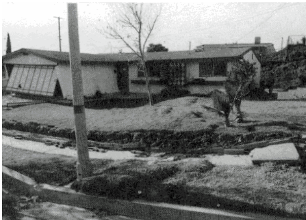
Large fissures in the ground, massive ground movement or slope displacement. Condition: AREA UNSAFE
