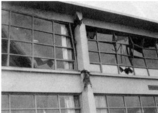
Obvious damage to primary structural elements, severe cracking of walls, or other signs of severe distress Condition: UNSAFE
